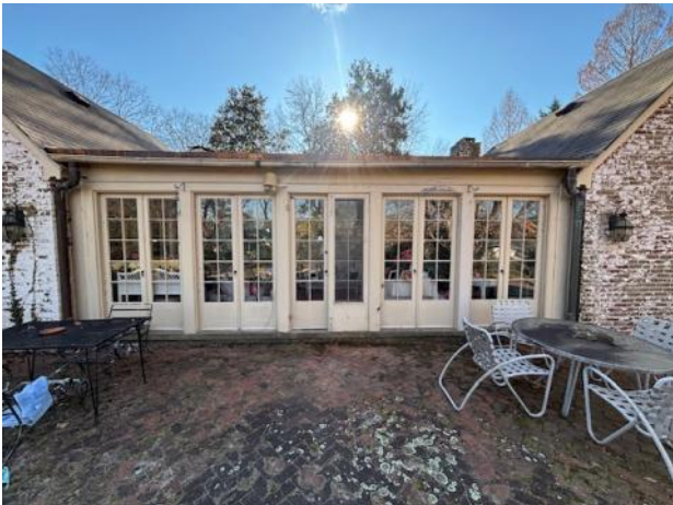
ENCLOSED PATIO - DOOR DAMAGE
