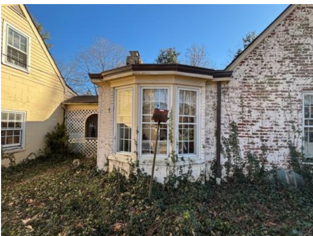
BAY WINDOW - ROT/DAMAGE
