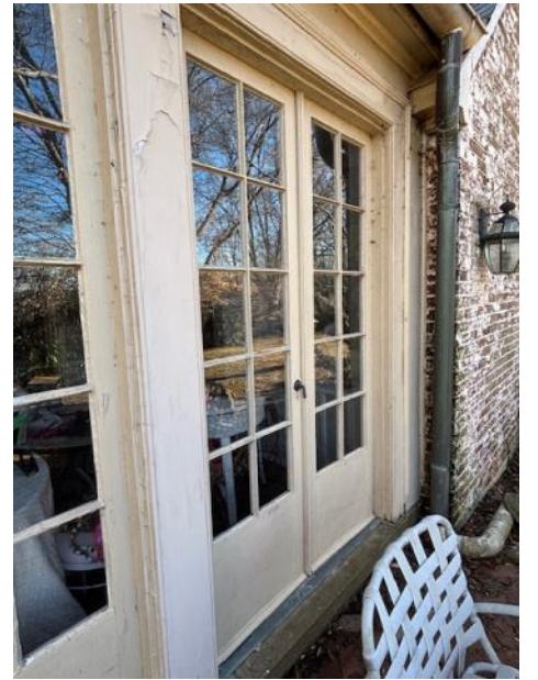
ENCLOSED PATIO - DOOR DAMAGE
