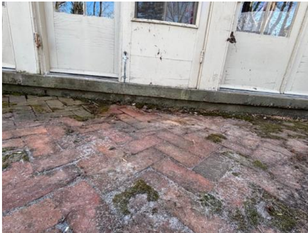
ENCLOSED PATIO - DOOR DAMAGE
